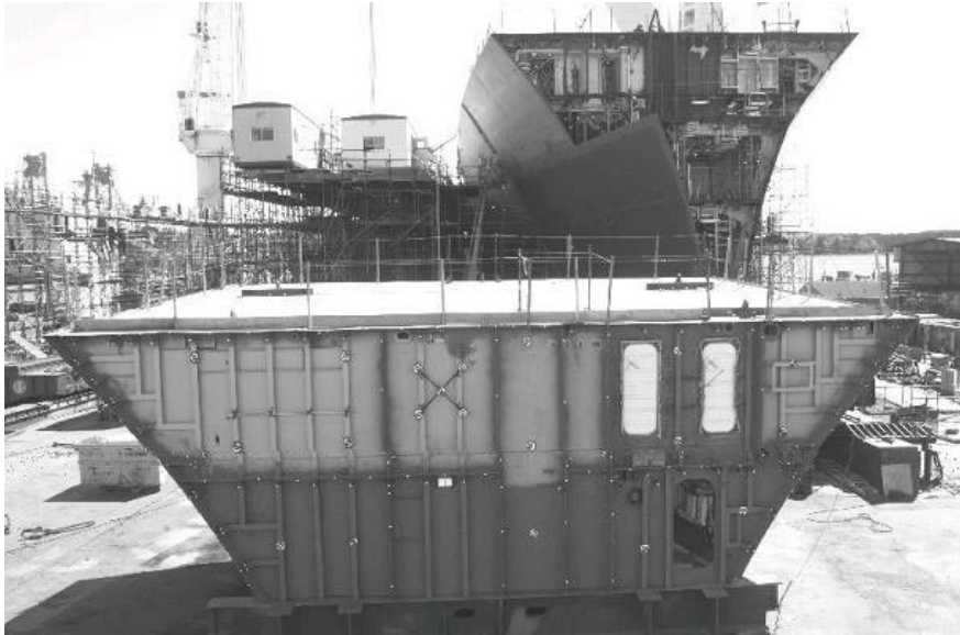
Figure A.1: A typical image of a ship bulkhead instrumented with retroreflective photogrammetric targets. The Imetric orientation cross is visible in the centre. Image courtesy of Bath Iron Works.
